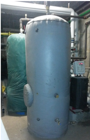
Figure 2 Insulated hot water storage and mixer
