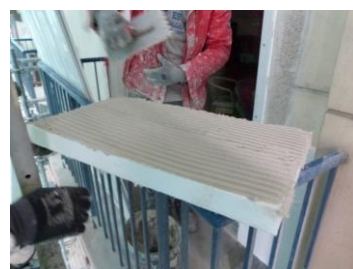
Figure 6+7 By installing an ultra-thin Aerogel insulation EIFS, the depths of the balconies will still allow to actually use the balconies with minimal loss of space. The system is the first of this kind to be installed in France.
