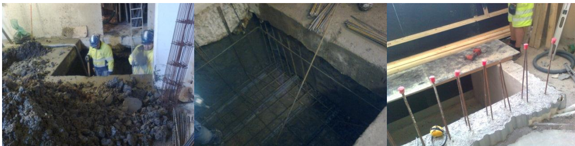
Figure 5 Some of the operations involved for elevator pits. Left: Excavating by hand inside a building. Center: Reinforcement on the gravel floor. Right: After excavation and casting of pit, House J
