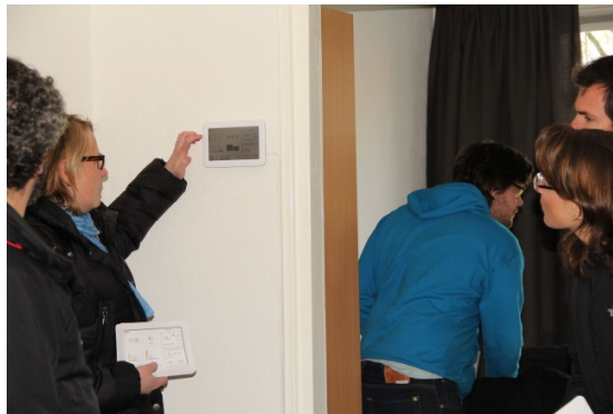
Figure 1 The Eneco Toon display installed in a dwelling. Source: Skanska
